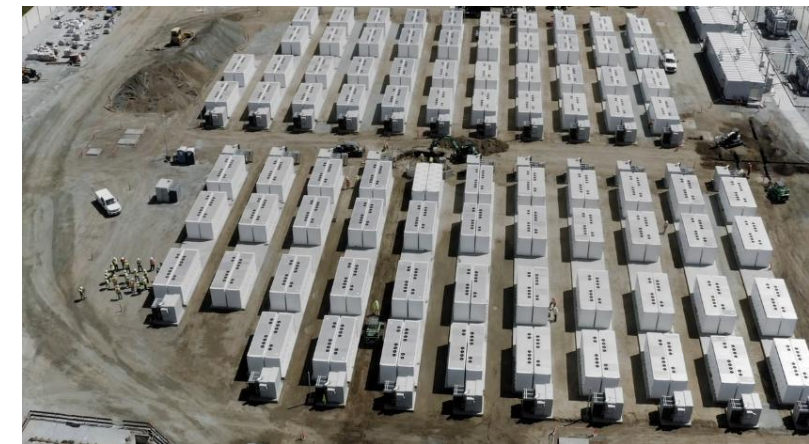
Tesla Megapacks, Moss Landing
