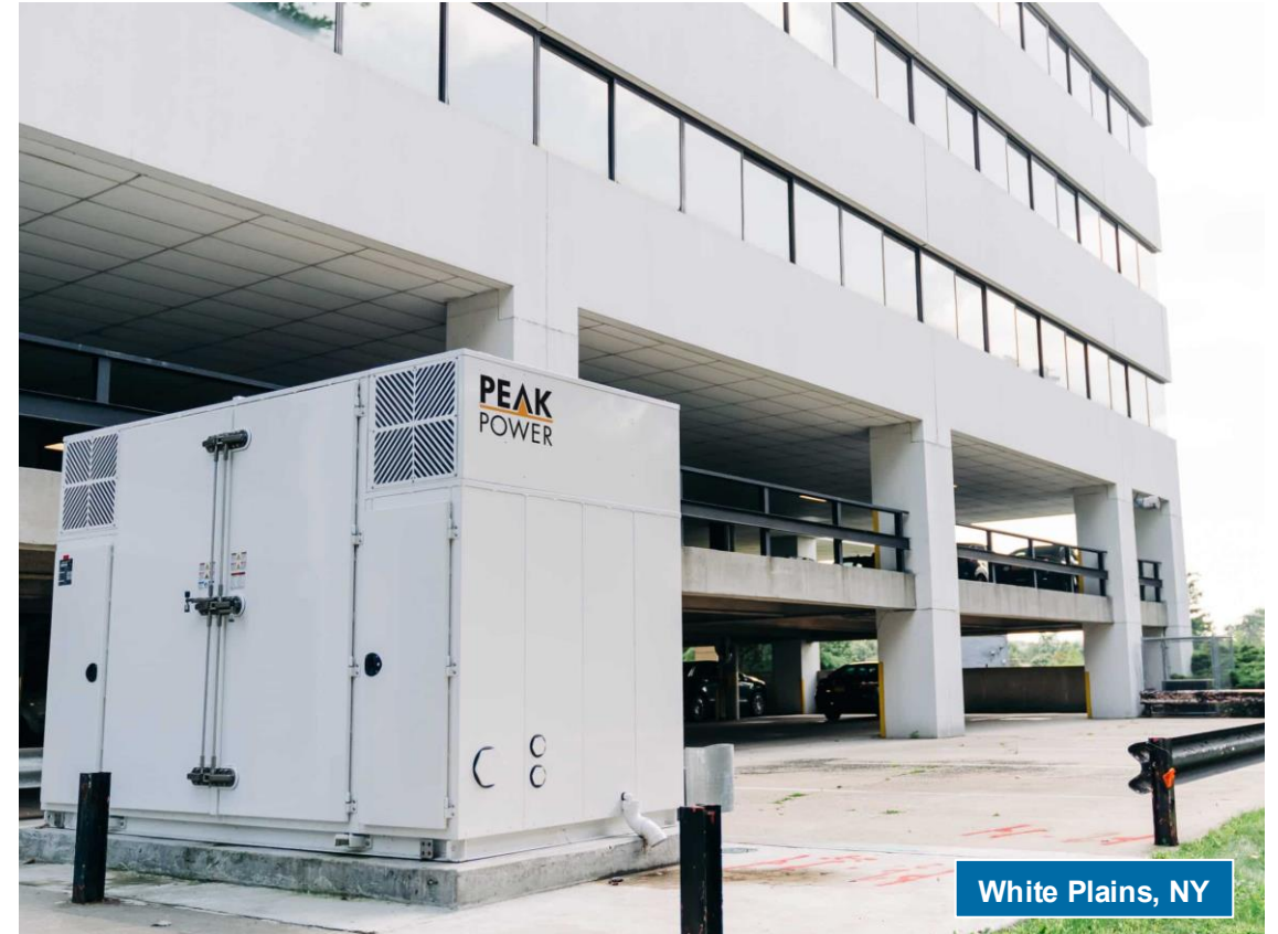
375 kW / 940 kWh installation: Peak Power project , part of a virtual power plant arrangement with Con Edison; sited at commercial office location in White Plains, NY.
