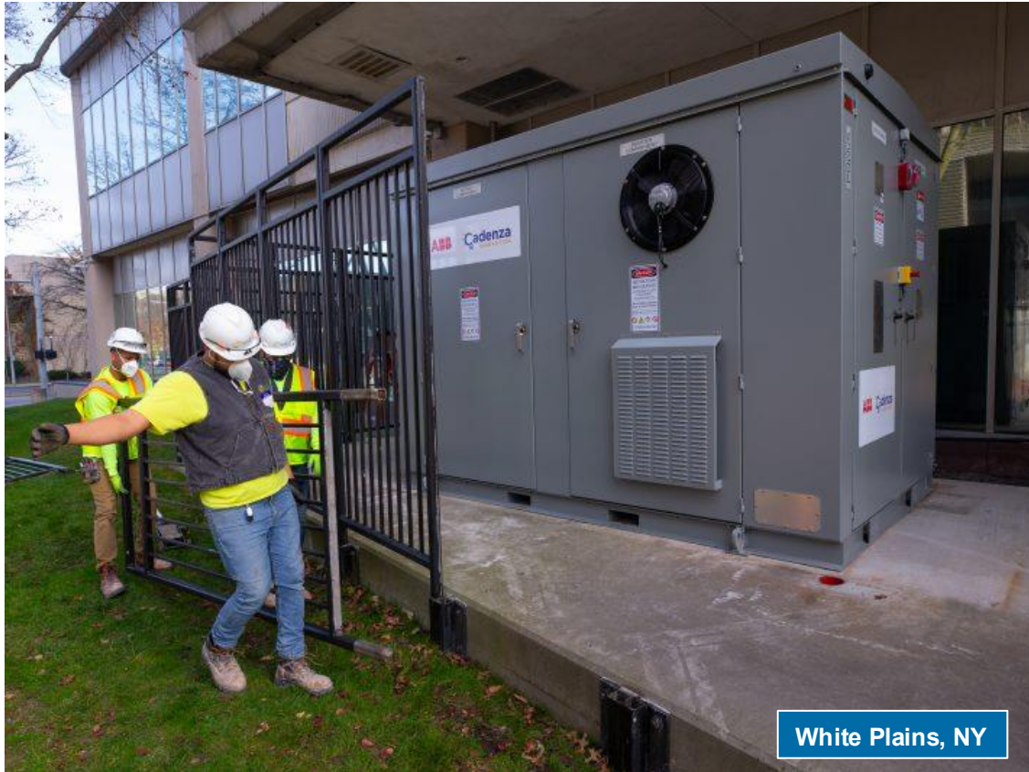
50 kW / 250 kWh installation: Cadenza Innovation system , in collaboration with NYPA and NYSERDA; sited at commercial office location in White Plains, NY.
