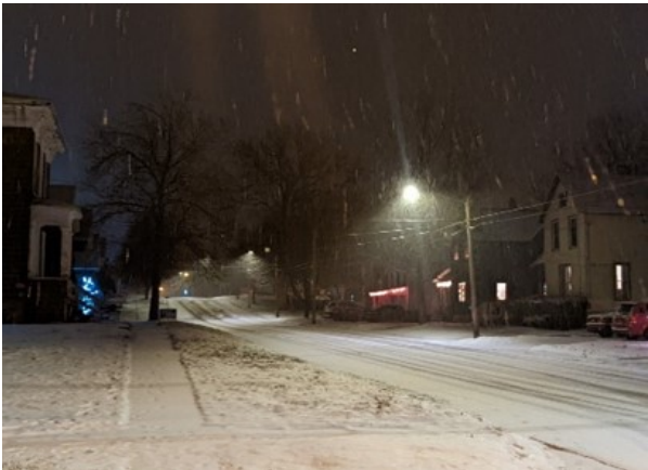
A newly installed LED streetlight casts light directly downward, improving illumination and reducing light pollution.
