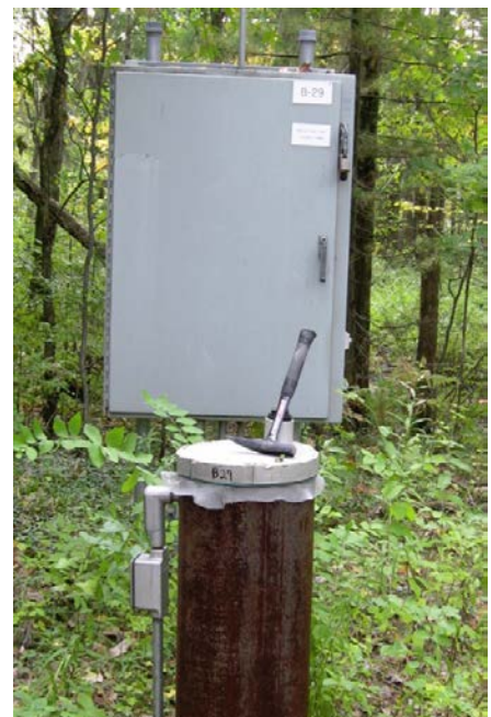
Continuous water-level and temperature data was recorded at specific wells. Well B-29 was in the Richland well-field.
